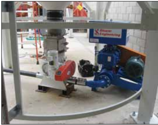
Blower Engineering equipment was used in the new grain screening and precleaning system, which was part of the grain storage expansion project. Photo by Adams Building Contractors.
