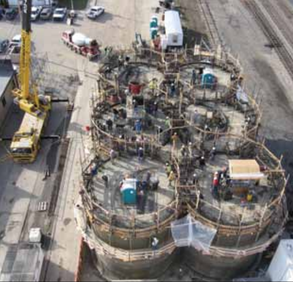
For 86 hours straight, concrete was poured into slipforms for the six grain storage silos at Chelsea Milling. Photo by Adams Building Contractors.
